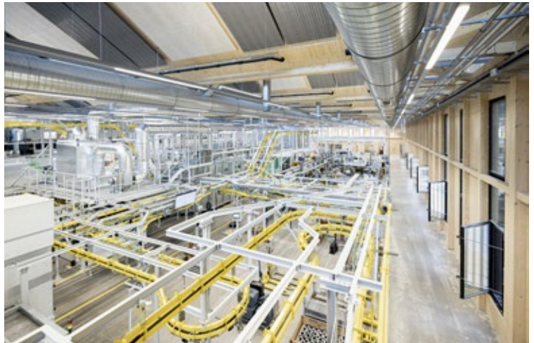
V-ZUG production hall with enamelling plant (high-temperature process) for ovens
