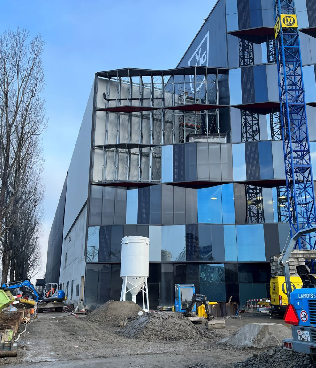
Installation of power facilities for the Multi Energy Hub in the existing "ZUGgate" warehouse building
